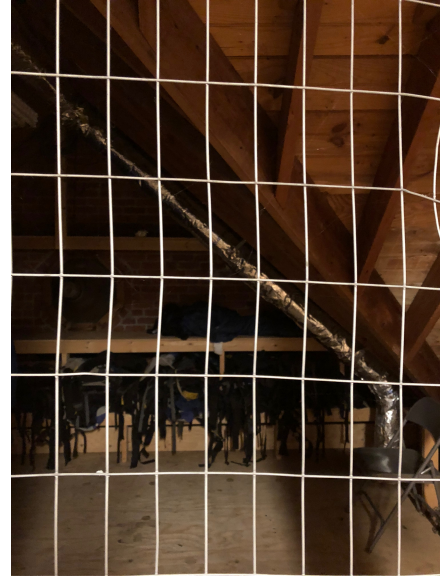
Figure 2.7: Ventilation Ducts in the Attic-2
