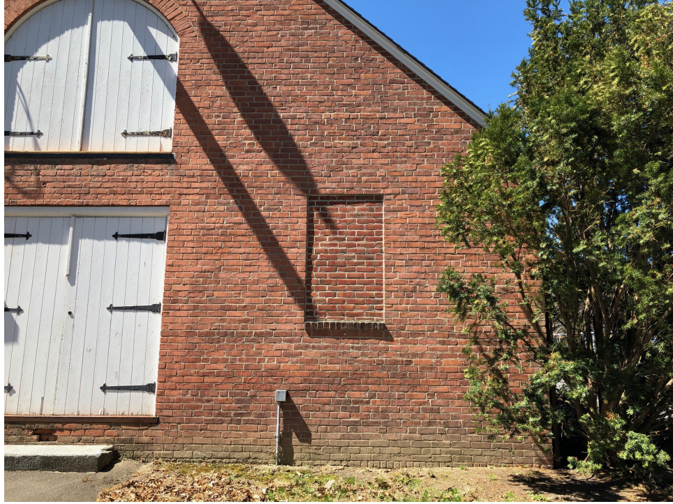
Figure 4.2: One of the Two Windows at the Field House that were Removed
