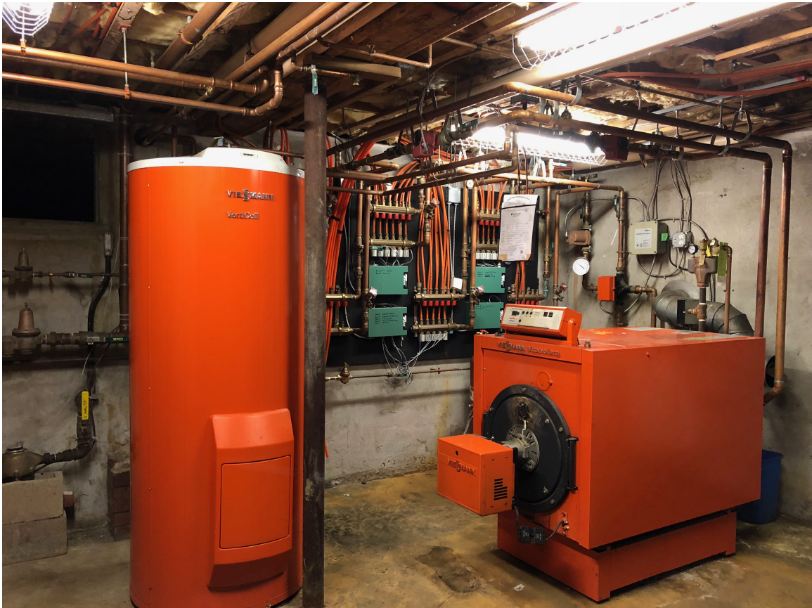
Figure 2.4: Boilers for Heating and Domestic Hot Water at the Basement of Field House.
