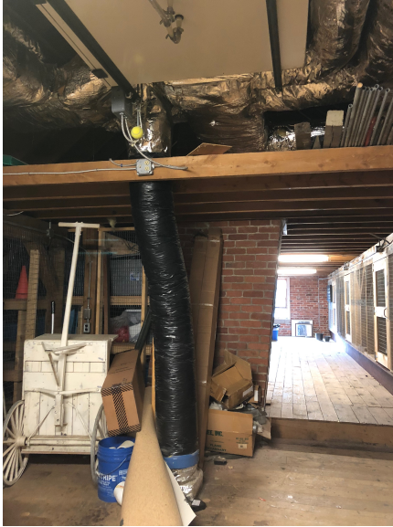
Figure 2.6: Ventilation Ducts in the Attic-1
